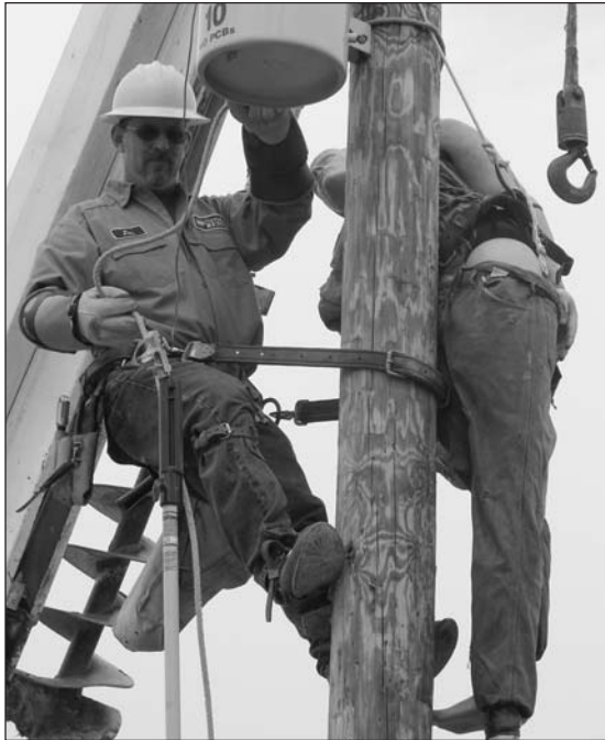
Lineman Jim Bischoff practices pole top rescue on a mannequin. This training is required for linemen annually. All linemen must complete a rescue within six minutes to meet the OSHA requirement. Although they practice to be ready in an emergency, linemen hope they never have to use this skill in an actual situation.
